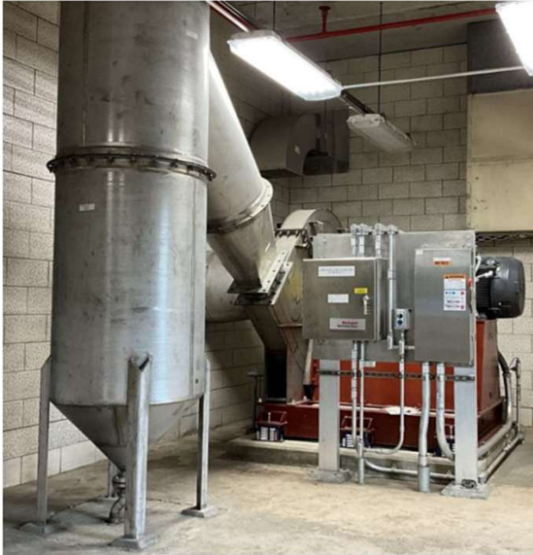
Induced Draft Fan
